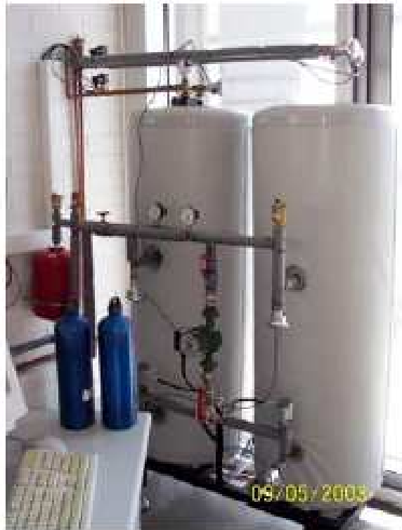
water tank with PCM modules inside
